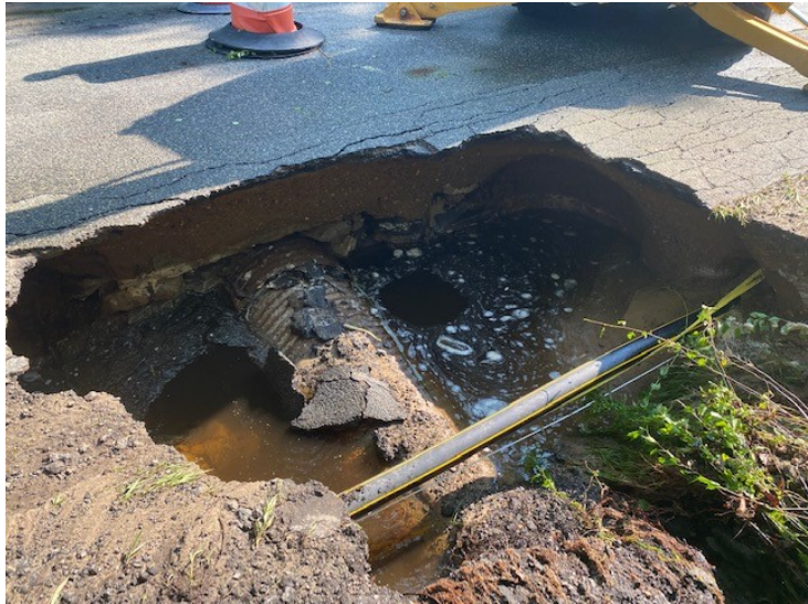
1 Lockwood Lane Culvert Failure
