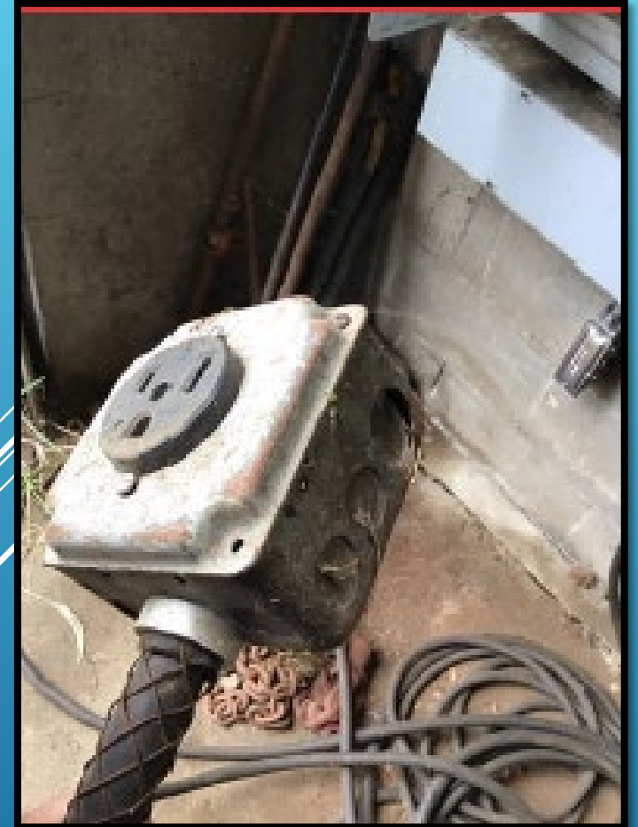
Poor ventilation, antiquated electrical & mechanical system
