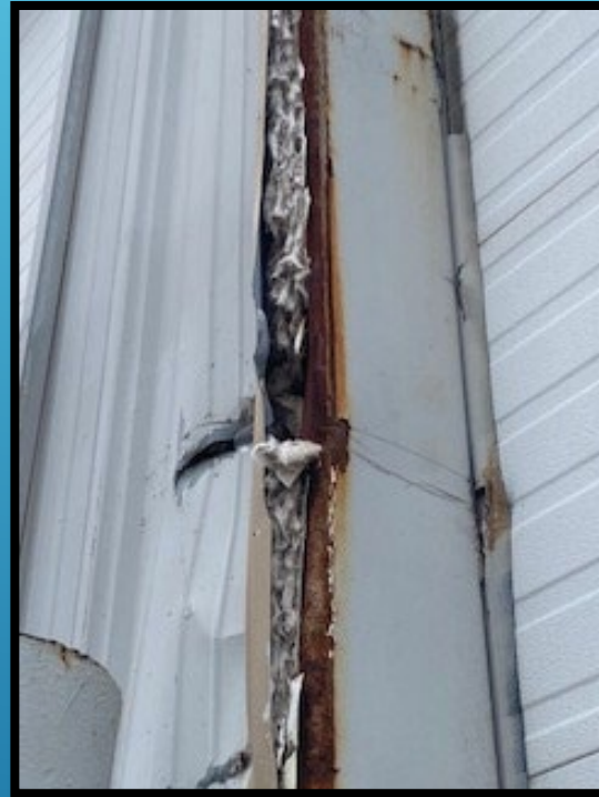
Rusted Sheet Metal Panels
