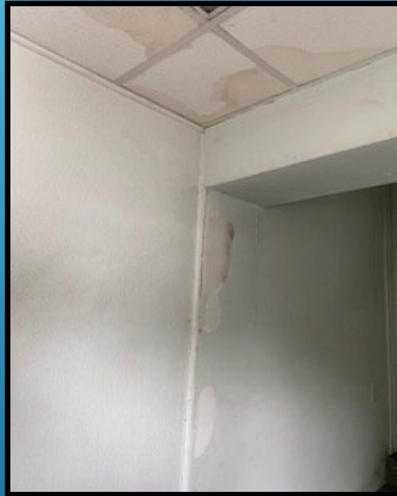
Water Leaks in Office Space
