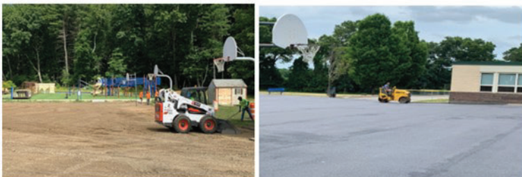
Before and after photos of recent paving project at Spofford Pond School.
