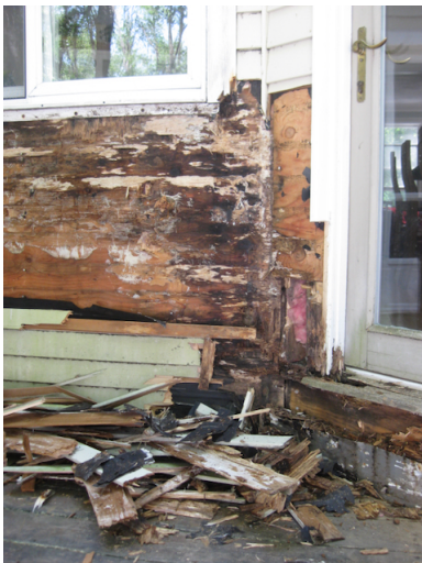
Tree canopy promoting rot from moisture
