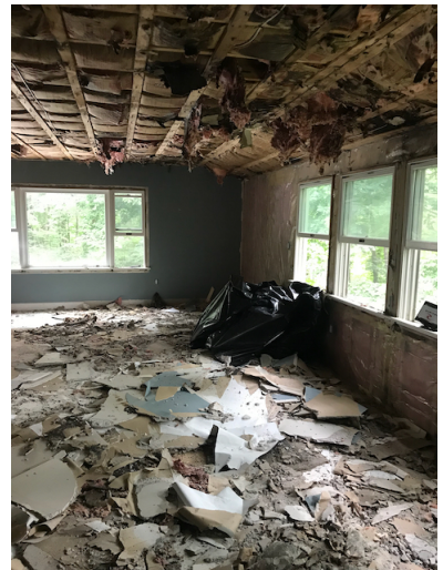
Tree damage to roof resulting in leak and requiring full gut and rebuild of room
