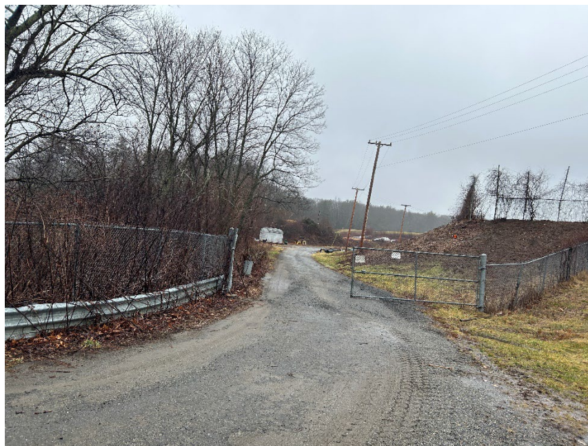
Figure 3 – Status of chain linked fence perpendicular to the DPW Access Driveway. As well as wooded areas along the eastern perimeter of the driveway. Photo taken facing southeast.
