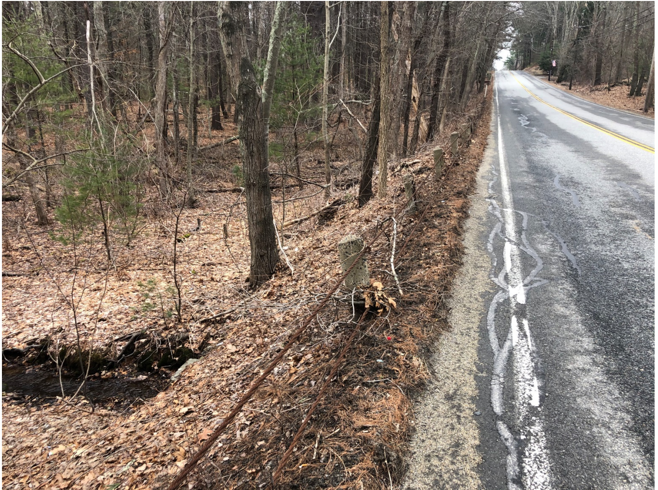
Figure 1: Culvert outlet on the north side of Willow Rd, photo taken facing east
