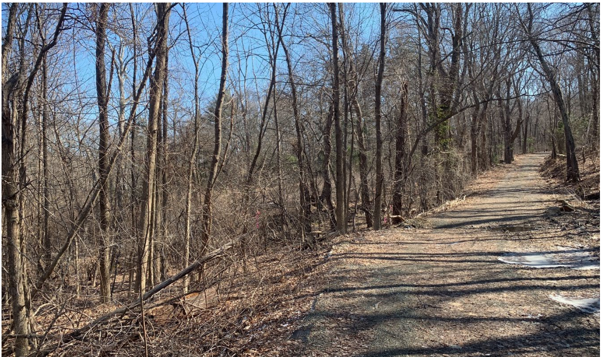
Photo #2: View of the access road by wetland series BO-W2. Erosion and rutting is visible along the access road in this location. Facing east
