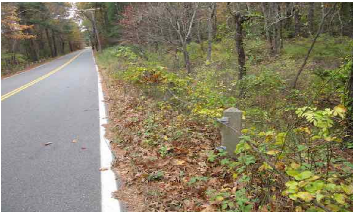
Photo G-1. Southerly view of guardrail adjacent to wetland G. Photo by B. Prokop 11/5/17.
