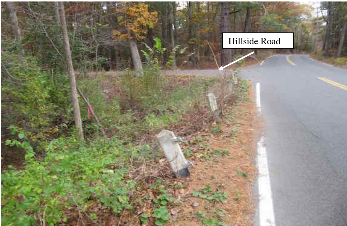
Photo G-2. Northerly view of guardrail adjacent to wetland G. Photo by B. Prokop 11/5/17.
