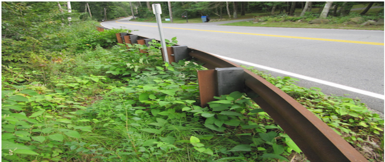
Photo B-2. Example of guardrail with corttel I-beam posts. Photo taken by B. Prokop on 09.17.18.
