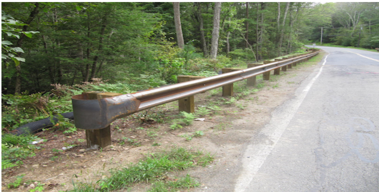
Photo B-1. Example of guardrail with pressure treated post. Guradrail installed off Middleton Road. Photo taken by B. Prokop on 09.17.18.
