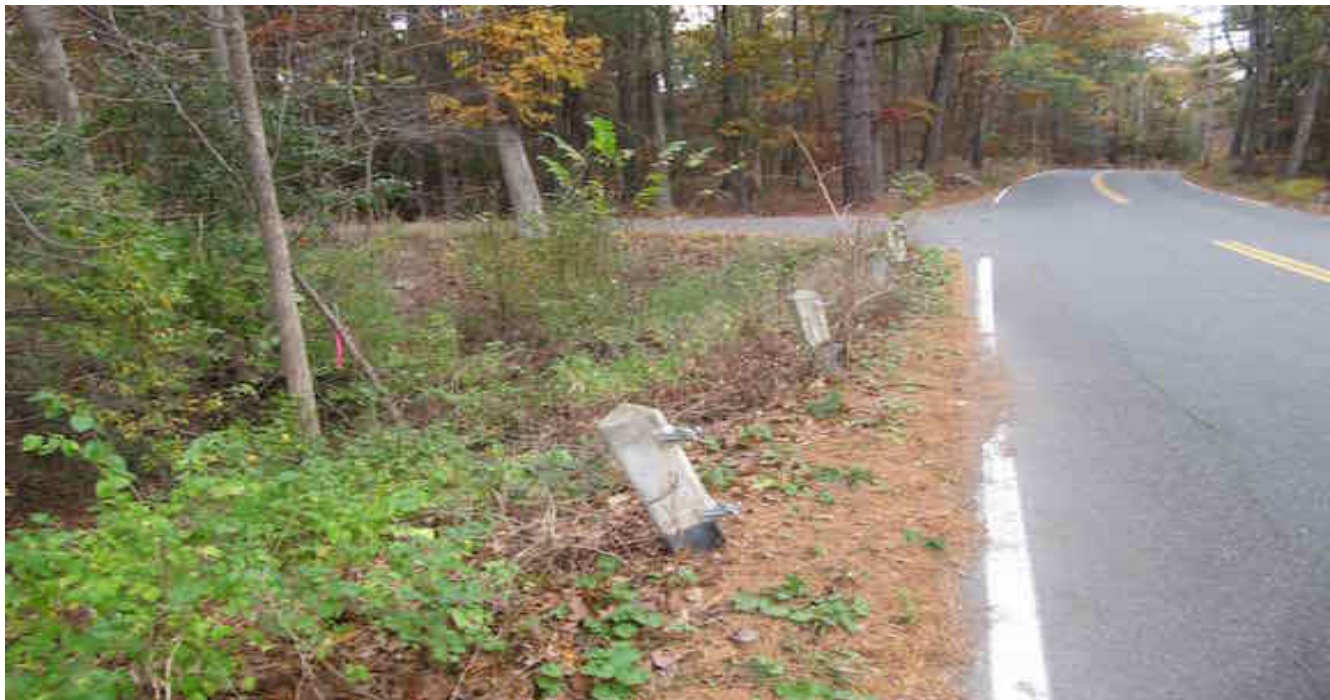
Photo A. Example of one of the eight guardrails proposed for repair and replacement. This particular guardrail is located on the western side of Georgetown Road just south of Hillside Road. The wetland with the “G” labeled flags lies at the road toe-of-slope. Photo taken by B. Prokop on 11/05/17.
