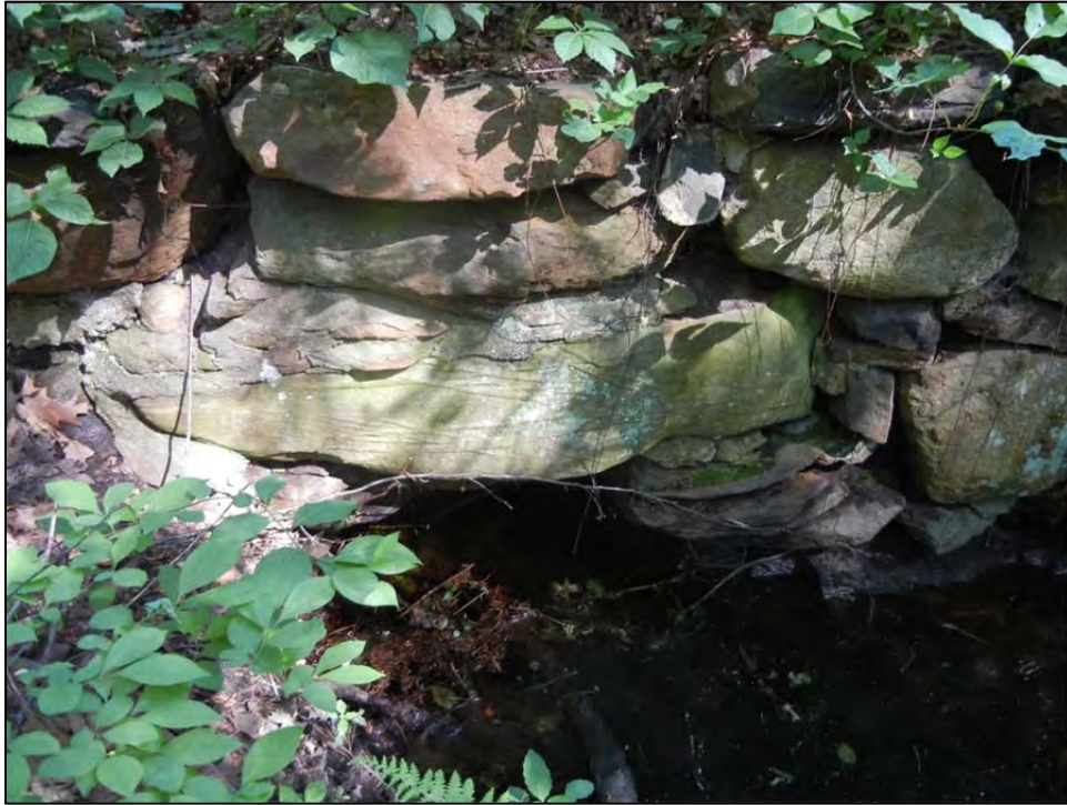
Photo No. 7 – 18-inch corrugated metal pipe downstream invert
