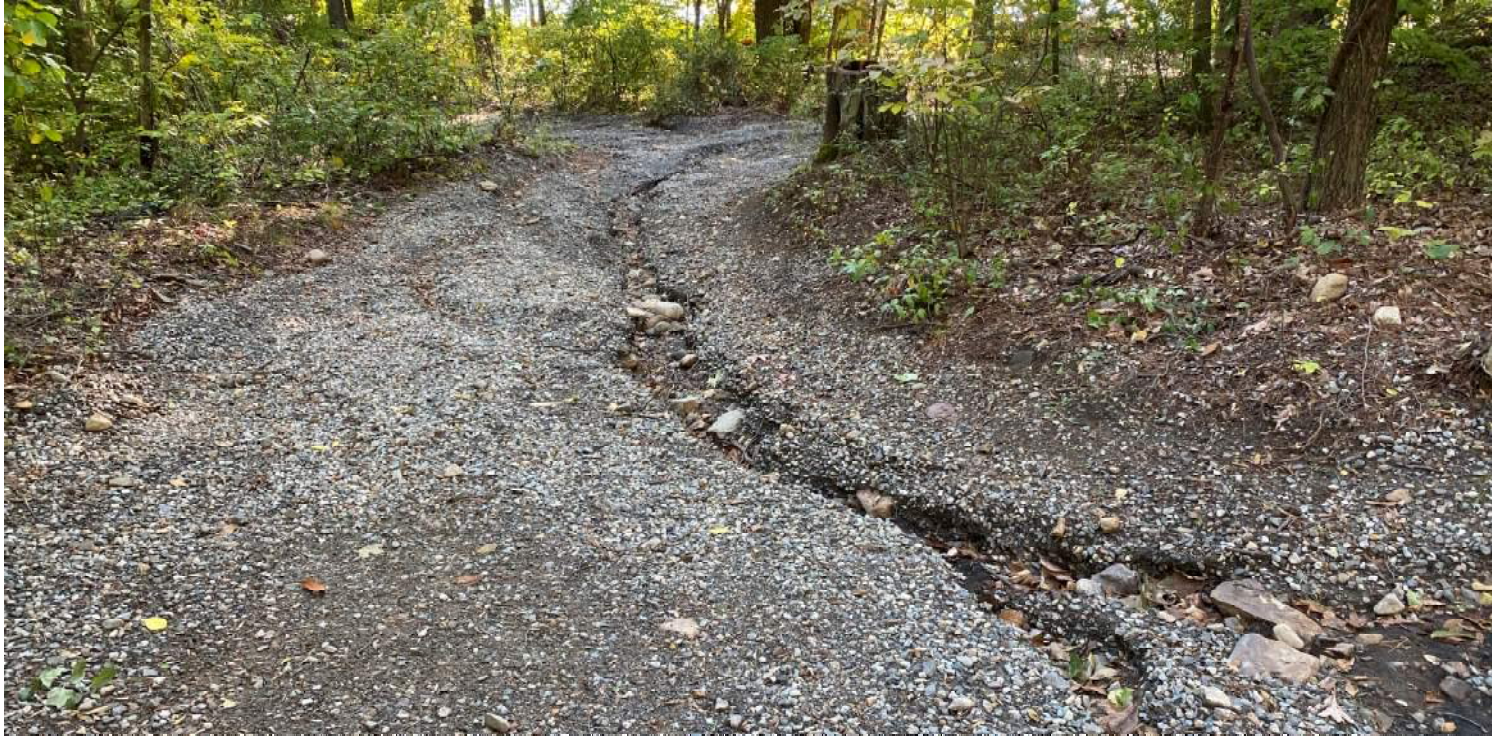
Photo #1: Existing condition of access road; severe erosion is evident in several locations. Facing South
