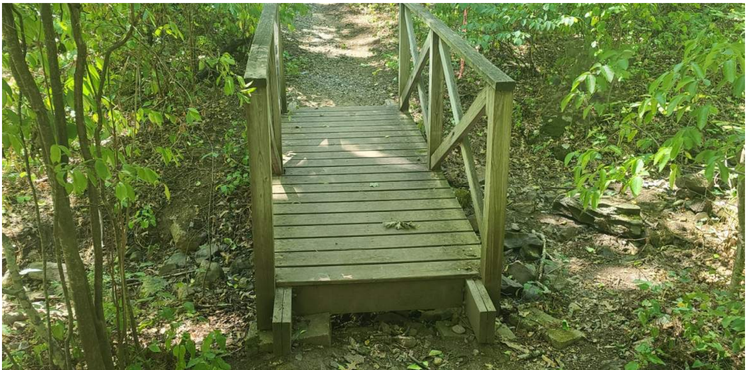
Photo #2: Undersized footbridge over intermittent stream to be upgraded for safety and accessibility. Facing East .
