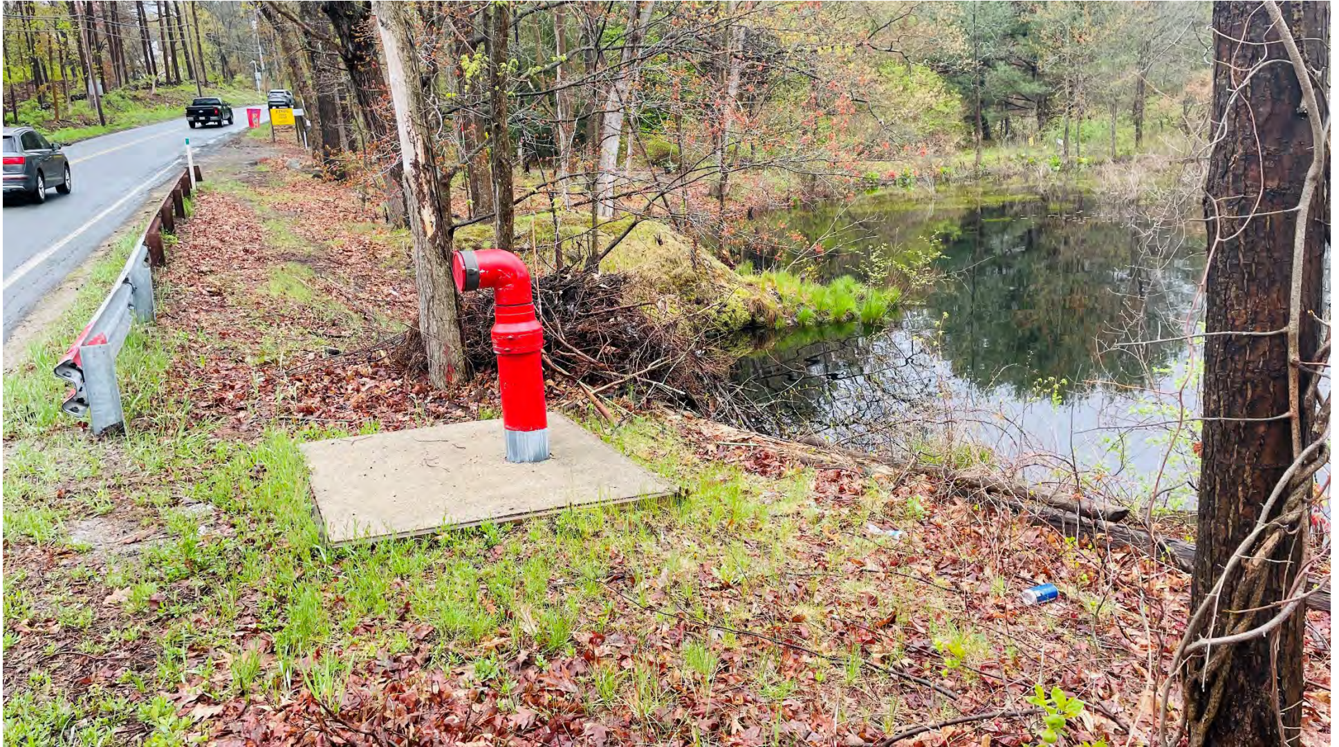
Photo 4 – Example of a dry hydrant located further upstream on the Parker River in Boxford, across from Boxford Animal Hospital.
