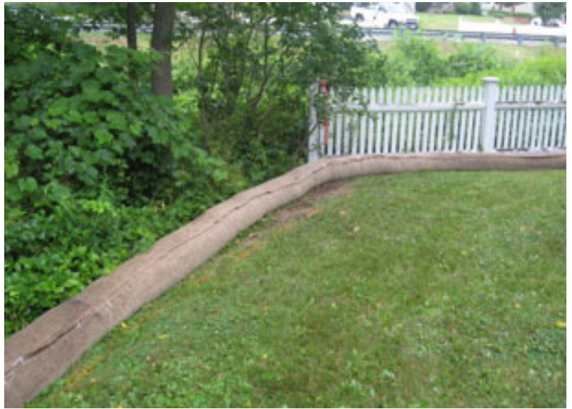
Example of the proposed siltation control barrier consisting of Groundscapes Filtermitt (12 or 18 inch tube) or equal
