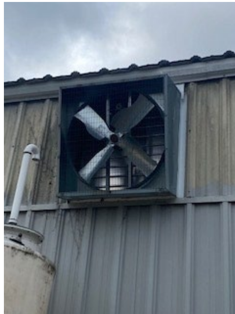
Ventilation Fan Never properly vented to the outside contributes to hazardous fumes within the building
