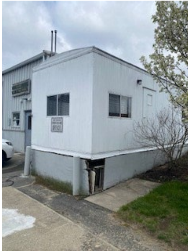
Rotting foundation attracts wild animals and causes excessive moisture/mold in the office trailer
