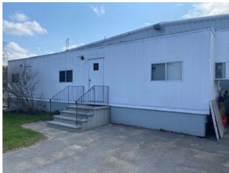
Office Trailer has no ADA Accommodations, Meeting Space Nor Adequate climate controls
