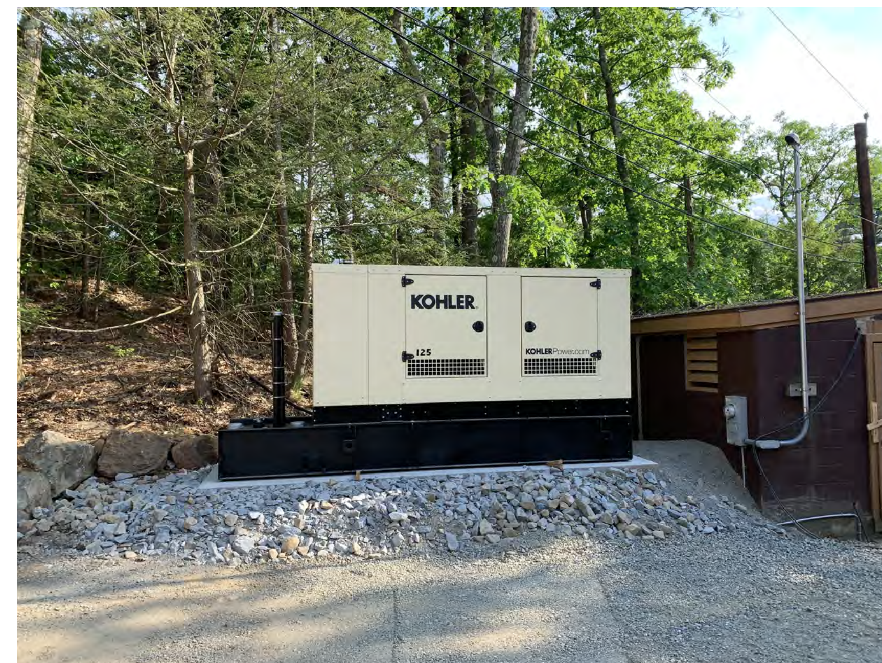
Generator relocated, left hand side out of buffer zone
