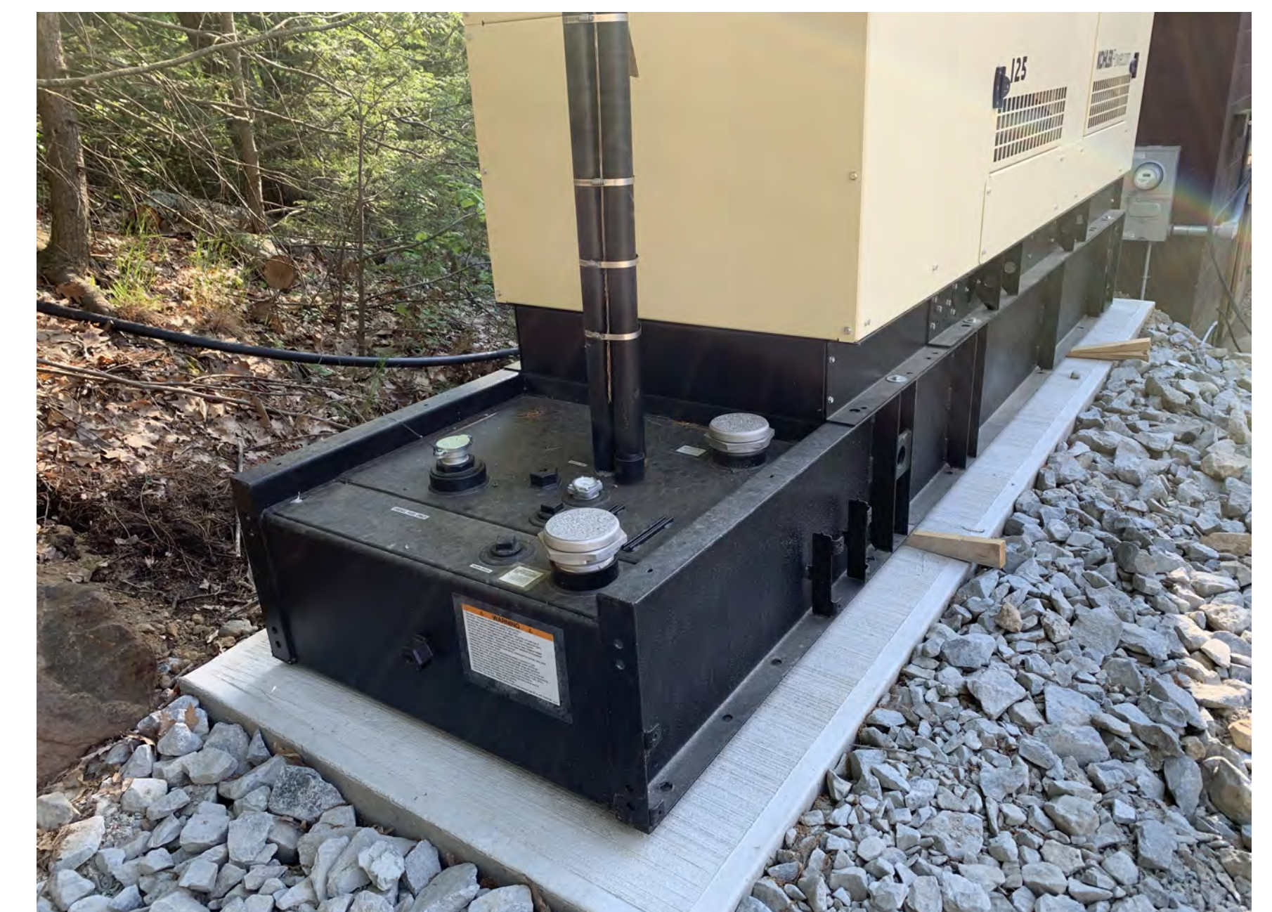
Close up of end of generator outside buffer
