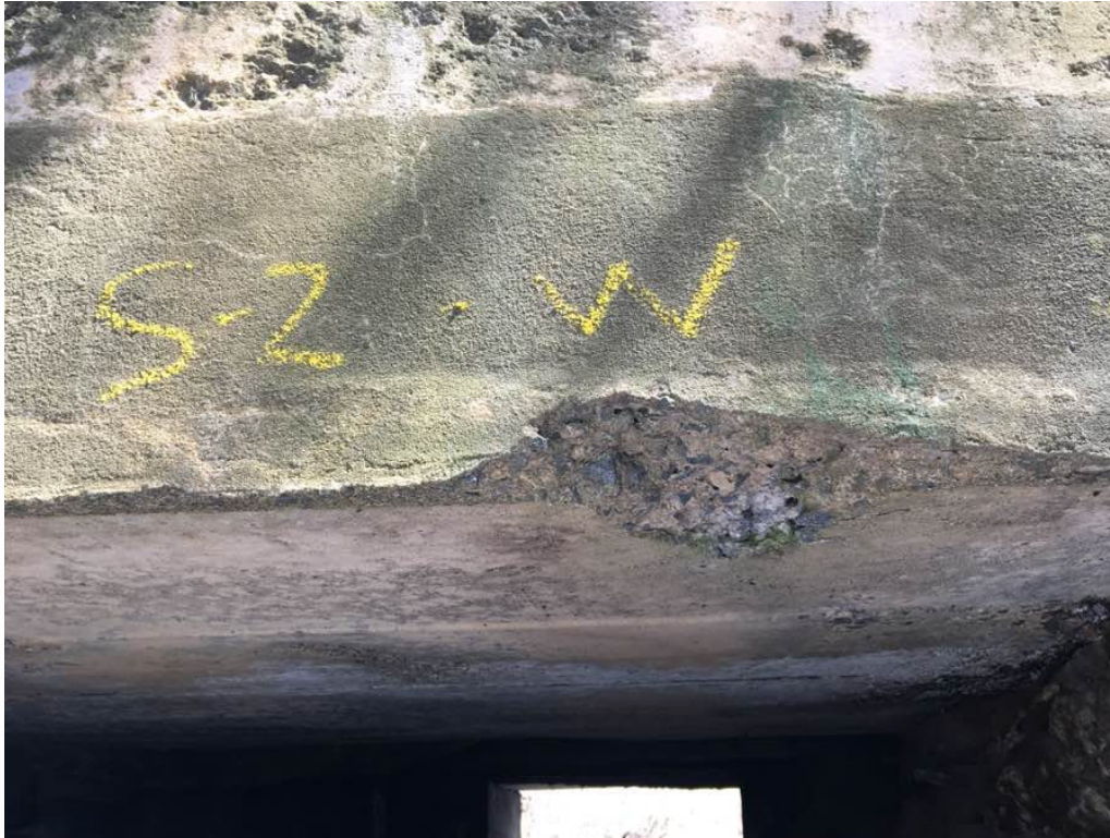
Photo 5: Span 2, spall up to 7" diameter at the edge of the west fascia.
