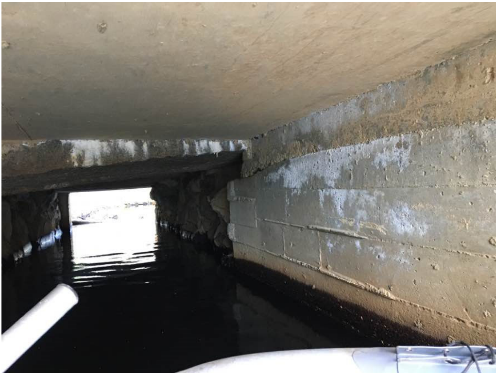
Photo 8: Typical abrasion along the water line and up to 2' high at the concrete walls. Also note the efflorescence at the east end of both north and south concrete walls. (Northeast wall shown).
