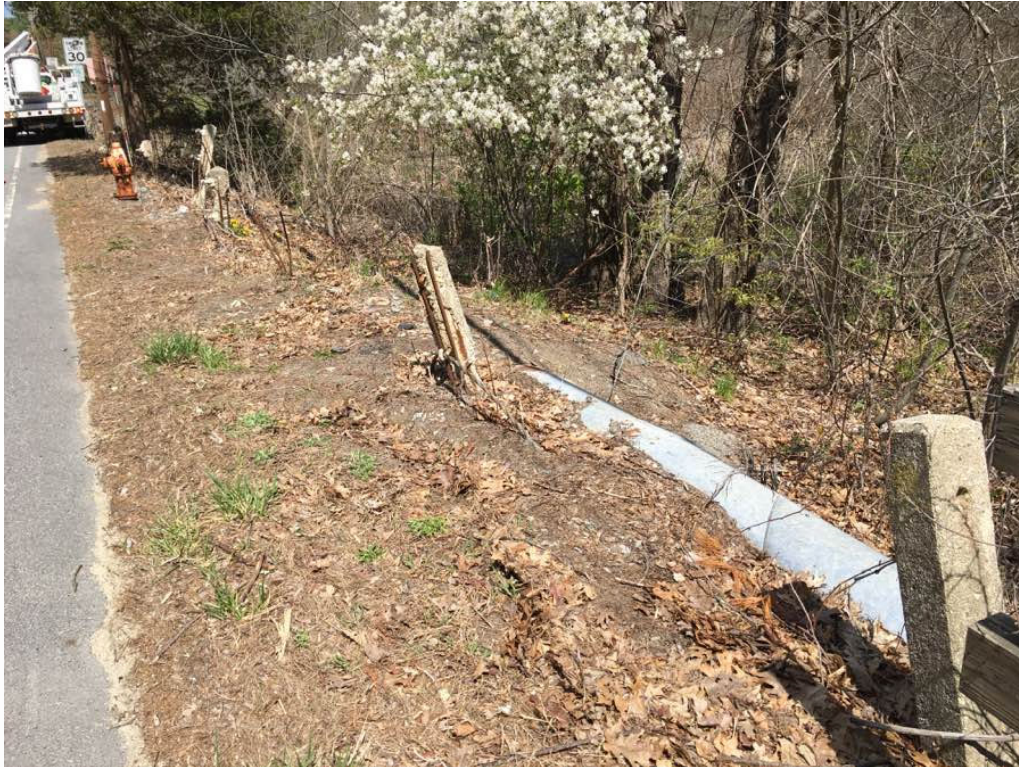
Photo 15: The northeast approach guardrail cables are missing, and the concrete posts heavily deteriorated and ineffective.
