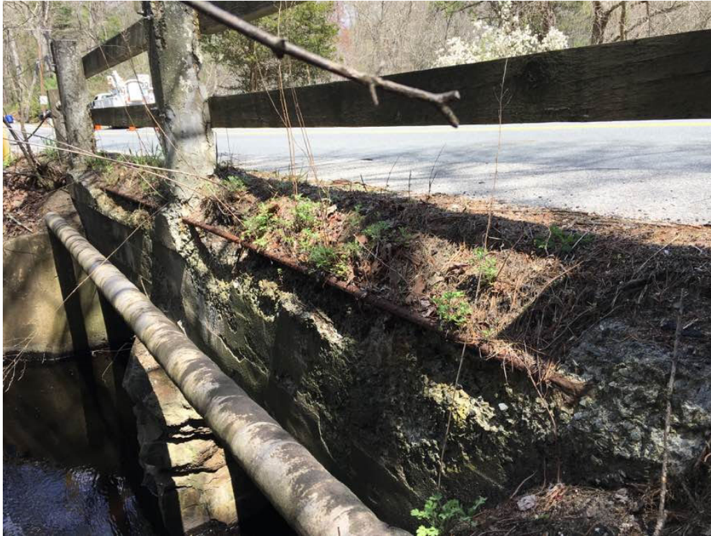
Photo 1: West fascia, areas of heavy and large spalls with exposed and rusted rebar.
