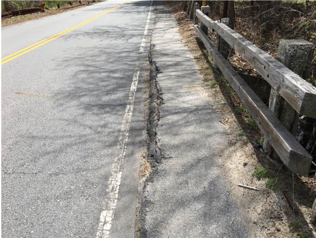
Photo 9: West sidewalk, deterioration at the curb which is propagating into the sidewalk.
