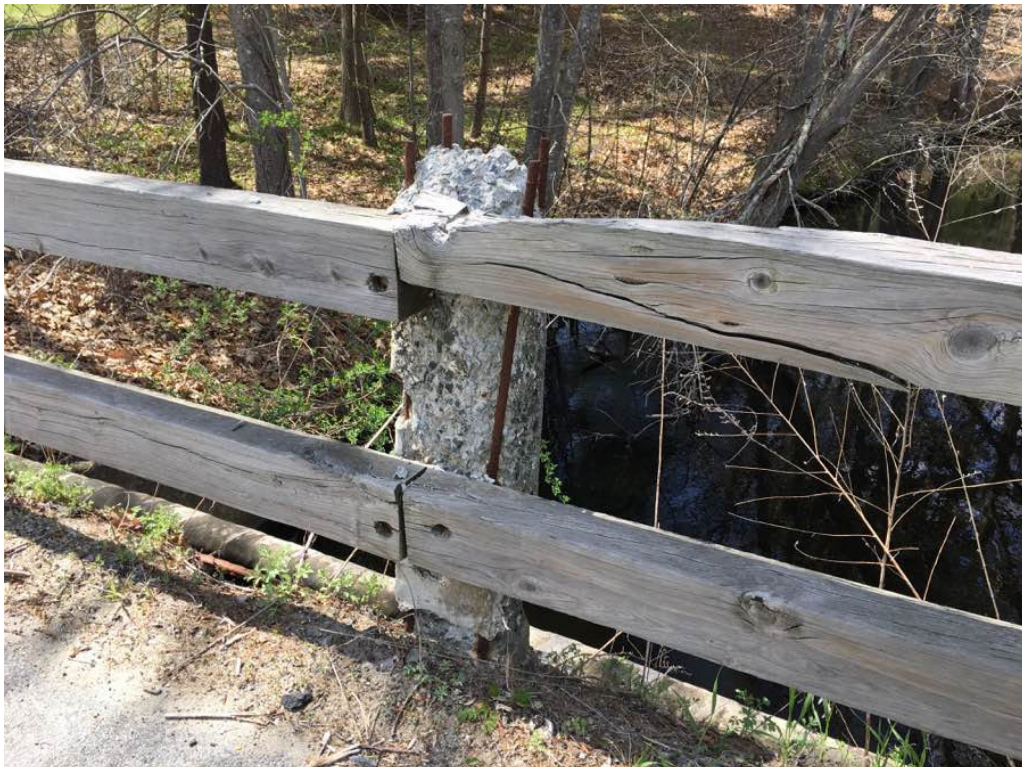
Photo 12: West bridge rail, the top rail has split and is not attached to concrete post. Also note the concrete post has heavy spalls with exposed rebar for the full height.
