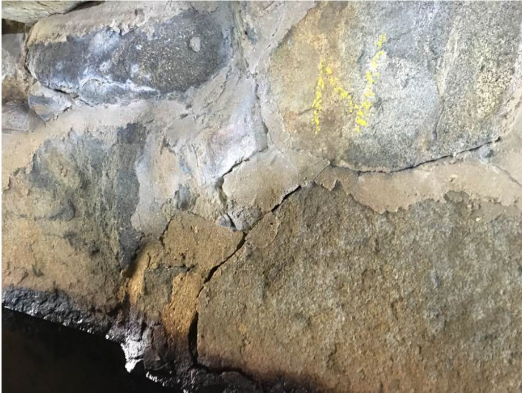
Photo 7: Typical cracking with efflorescence in the mortar between stones at all granite walls.
