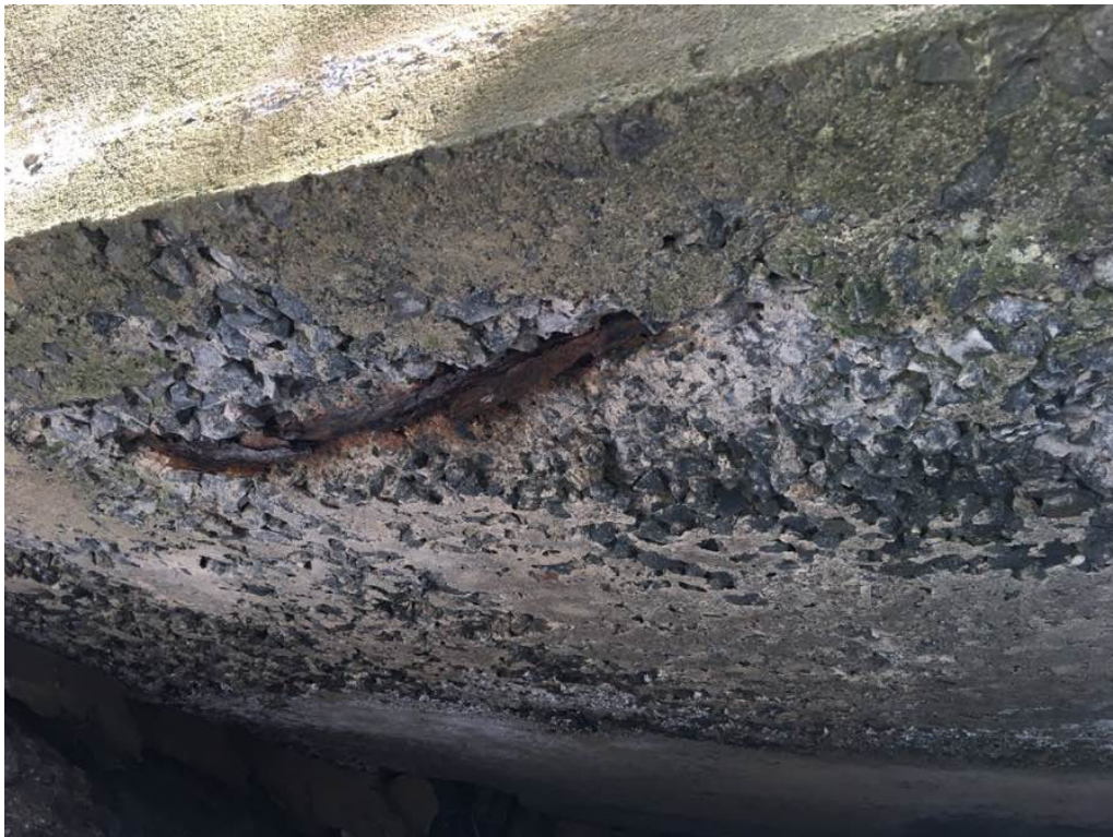
Photo 2: Span 1, near the west fascia, area of scaling, honeycombing and a spall at the concrete deck with exposed and rusted rebar.
