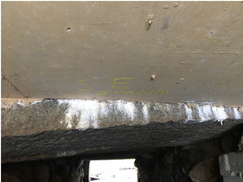
Photo 4: Active leakage with heavy efflorescence at the joint between the concrete slab and the first granite slab in span 1, near the east end.
