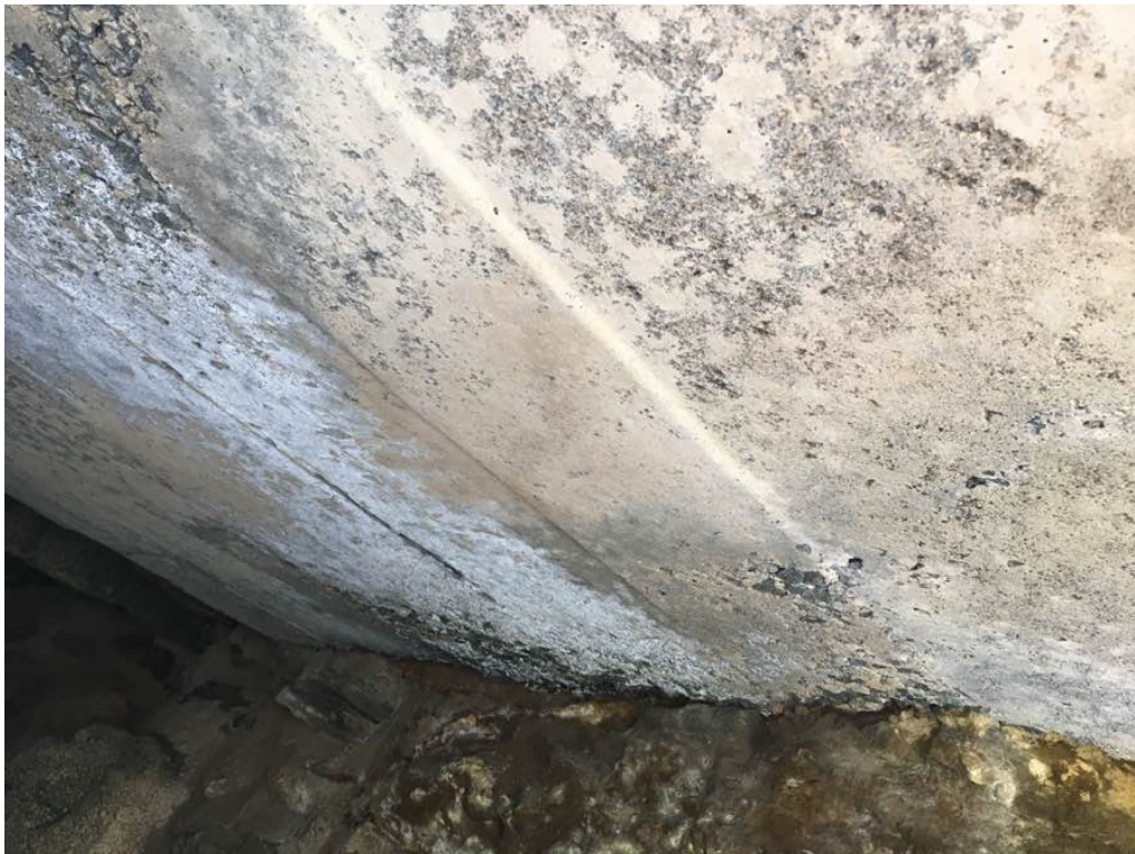
Photo 6: Span 2, west end, the underside of the concrete deck has full length x full width area of honeycombing/scaling with moderate efflorescence.
