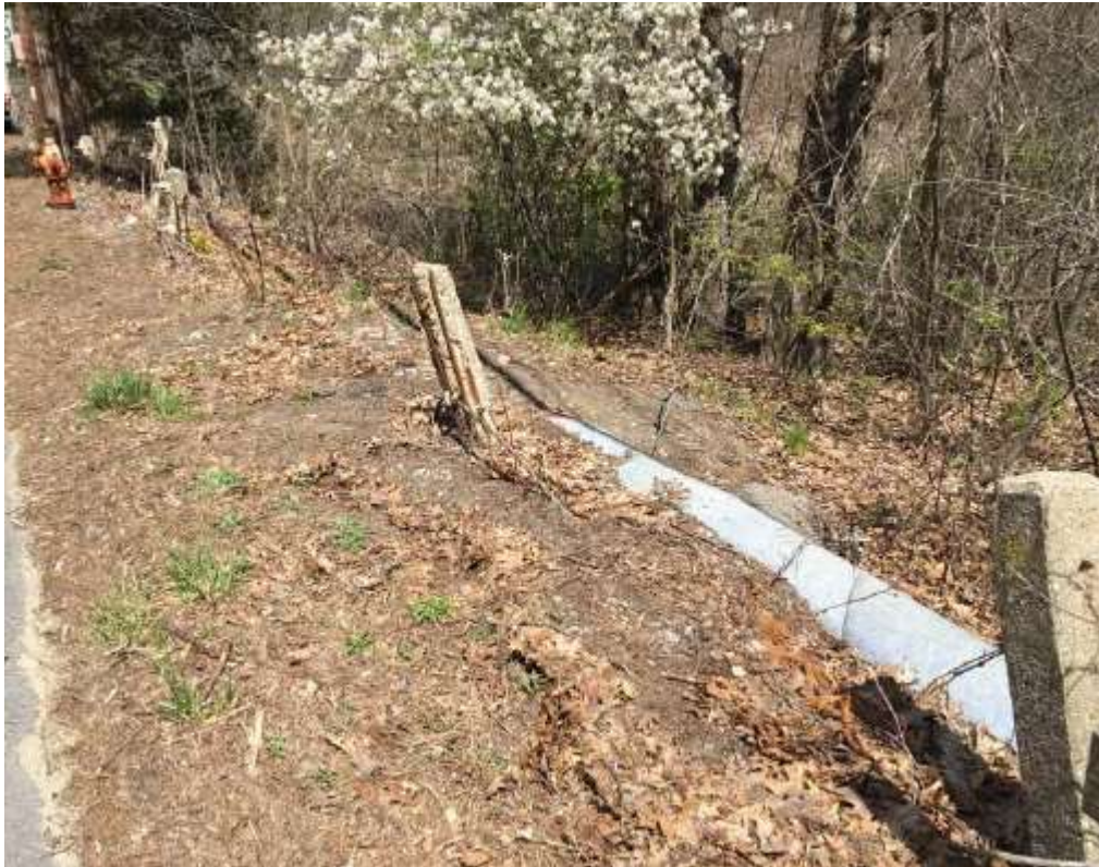
Photo 4: Northeast approach showing substandard traffic safety features (typical)
