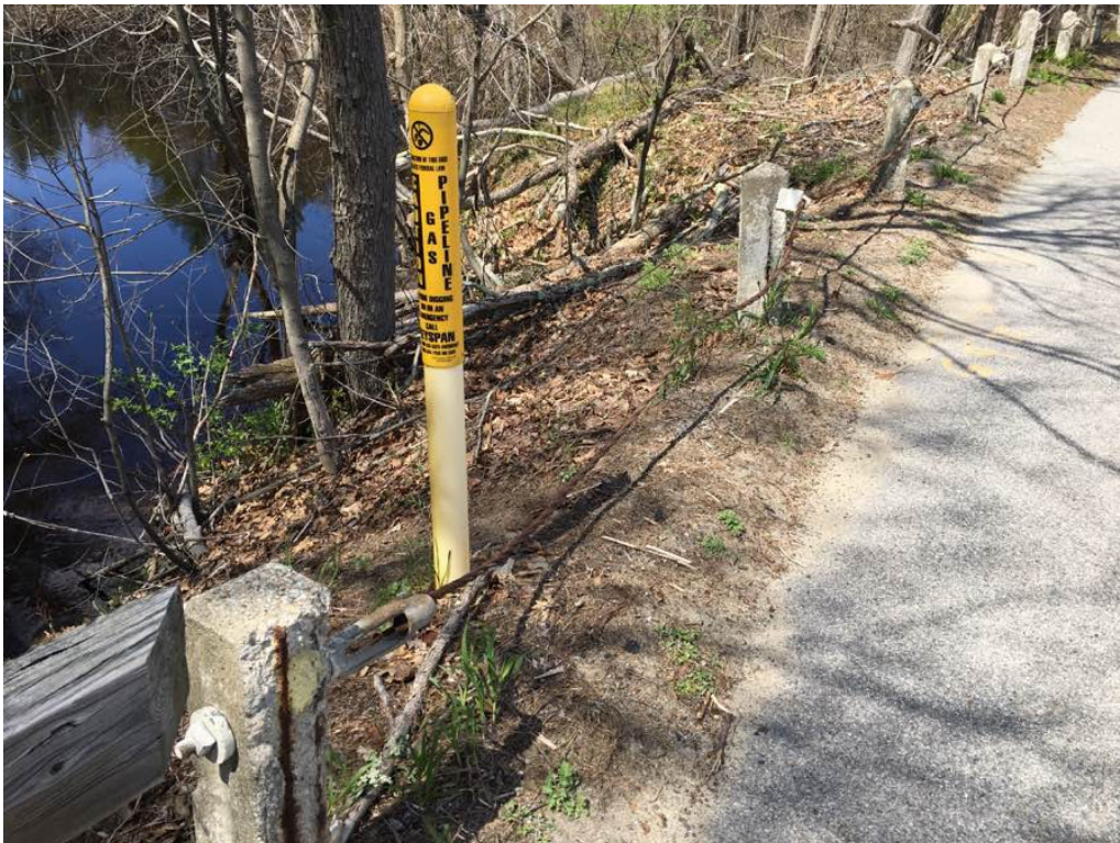
Photo 14: The northwest approach guardrail lower cable is missing, the upper cable is loose and ineffective and the concrete posts heavily deteriorated.
