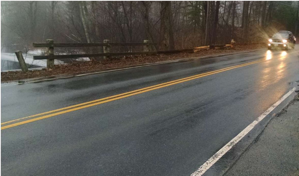
Photo 2: General topside looking west, note poor condition of sidewalk
