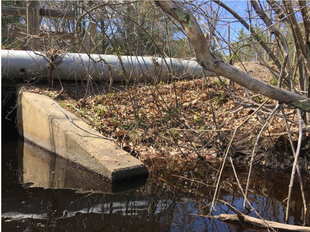
Photo 11: Minor erosion behind the northeast wingwall.
