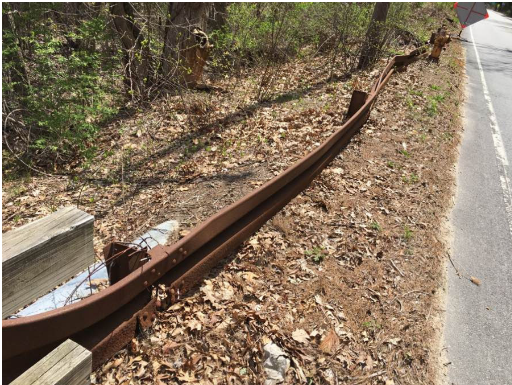
Photo 16: The southeast approach steel guardrail has 100% section loss, major impact damage and is ineffective.
