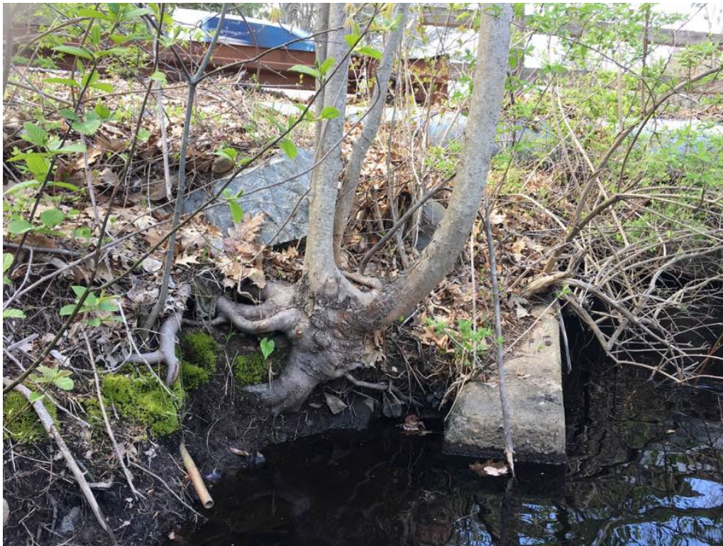
Photo 10: Minor erosion behind the southeast wingwall.
