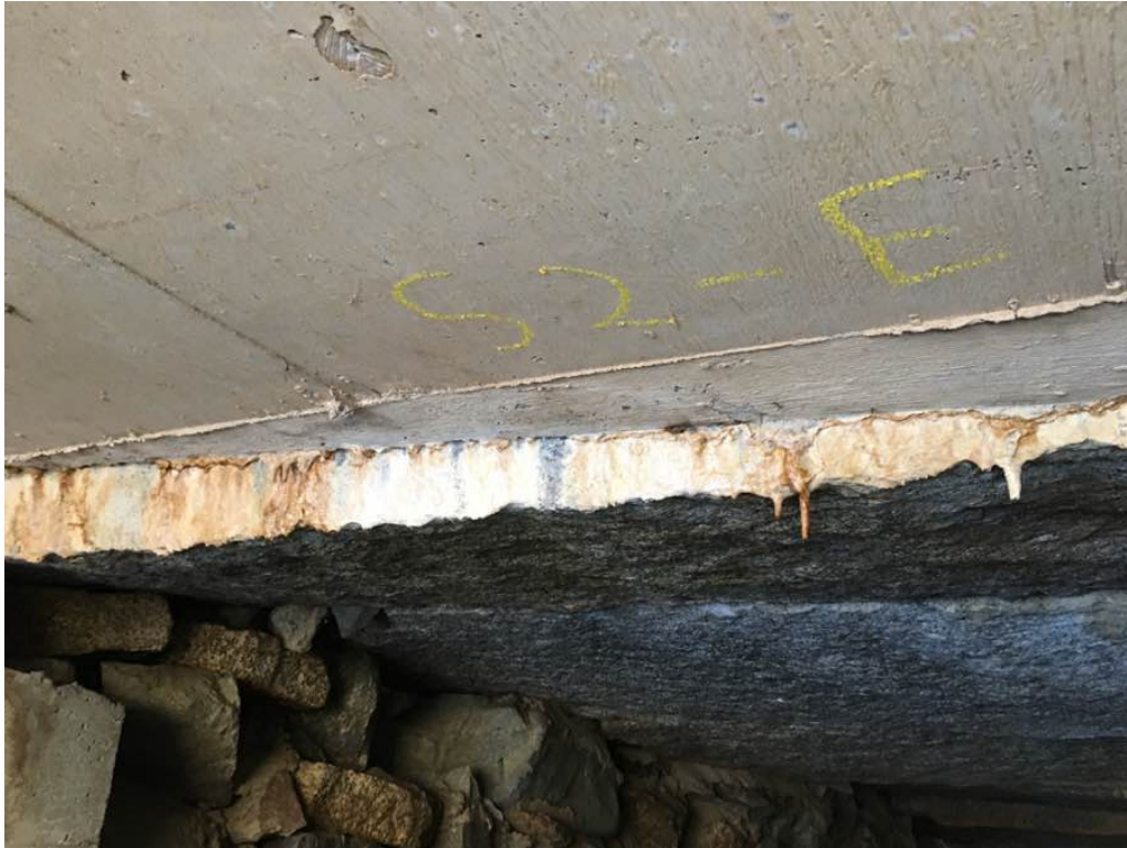
Photo 3: Active leakage with heavy efflorescence at the joint between the concrete slab and the first granite slab in span 2, near the east end.
