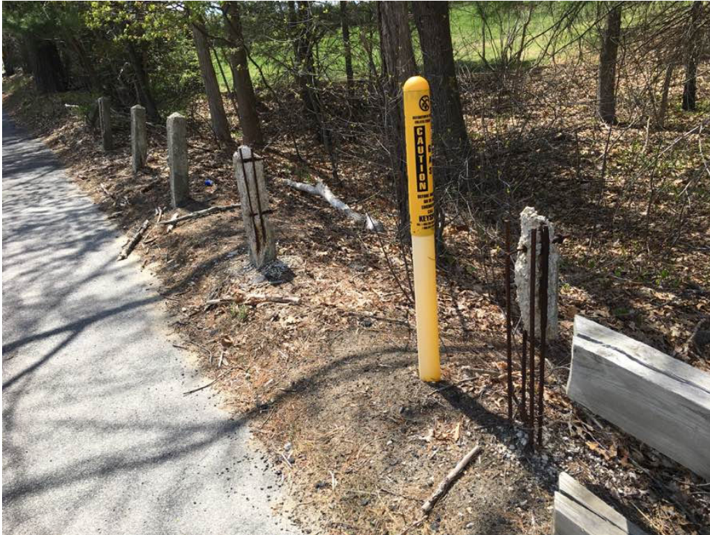
Photo 13: The southwest approach guardrail cables are missing, and the concrete posts heavily deteriorated and ineffective.
