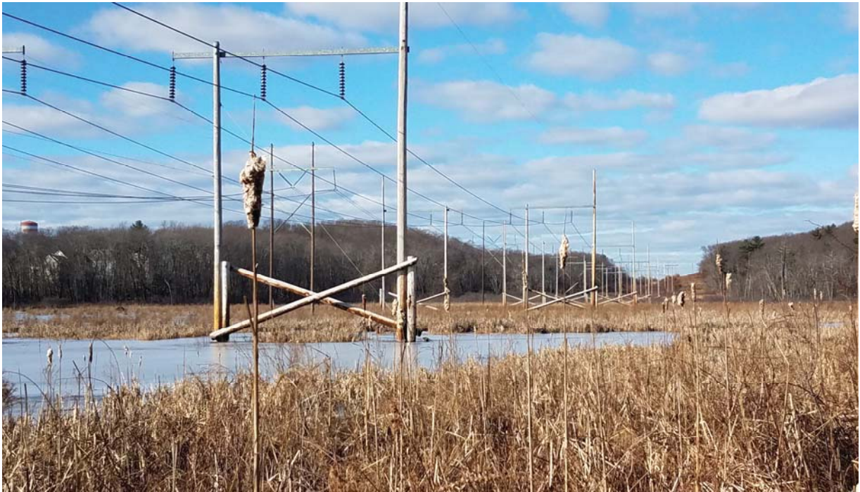
Photo 3: View of access road on the 394 Line off Washington Street. Facing north.
