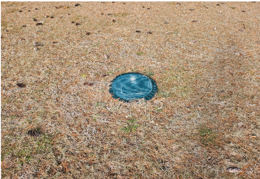
Photo #6: Location of newly installed septic system cover. Photo taken by Hancock Associates Staff Scientist on February 7, 2024.
