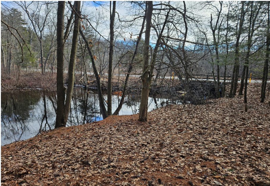
Photo #10: Bank of Fish Brook with view of culvert under Washington Street/Endicott Road located along the eastern edge of the property. Photo taken by Hancock Associates Staff Scientist on February 7, 2024.
