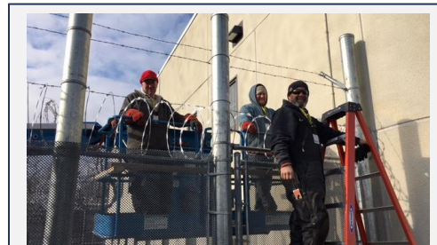
As part of the 80 Bed work, Northern Construction orchestrated fence repair work.
